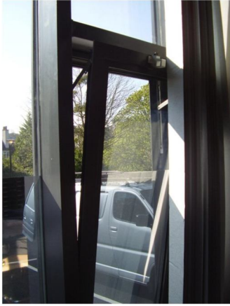
Figure 6.2 Example of ventilation area reduced by the restrictor. Column prevents window opening
